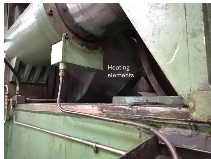
Figure 23. Heating elements of the rotocure
